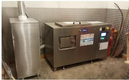
Site: Ahold Supermarket Location: Tabor, Czech Republic Machine: GG30s Install Year: 2016
