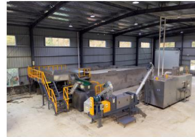
Site: Jiangle Composting Facility Location: Fujian Province, China Machine: GG500s Install Year: 2016
