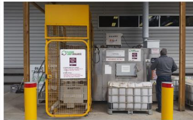
Site: Barwon Health Hospital Location: Geelong, Australia Machine: GG100s Install Year: 2013 Publications: The Fifth Estate June 2014
