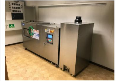
Site: Fazer Food Services Location: Stockholm, Sweden Machine: GG50s Install Year: 2017
